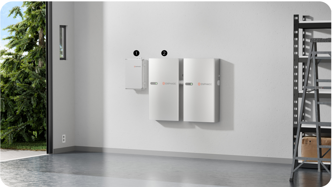
Figure 2: Wall-mounted, grid-tied system ① IQ Combiner ② IQ Battery 5P
