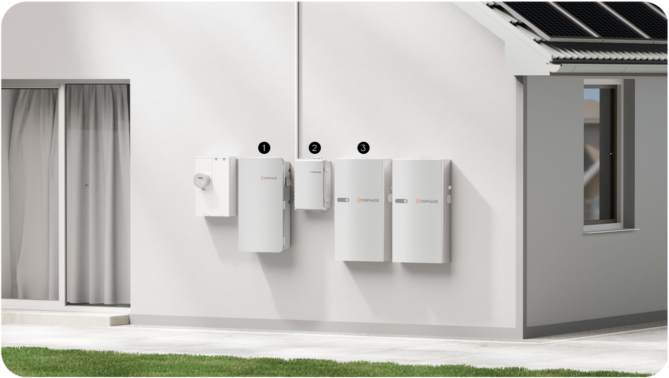
Figure 1: Whole home backup ① IQ System Controller ② IQ Combiner ③ IQ Battery 5P
